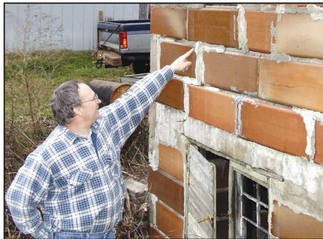
Peter Jacobs points out grout on the back wall of his sewer pipe garage. - photos by Ruth Nerhaugen
